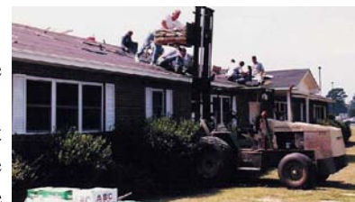
A much needed roof is installed on the Little People's dorm at the Children's Home by workers from White Savannah FWB Church, Oak Grove FWB Church, and North Conway Church of God
